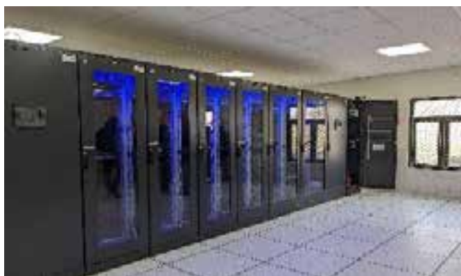
Image: New Data Centre at Sohra Campus
